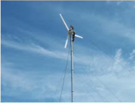
Wind Turbine / Turbin Angin
